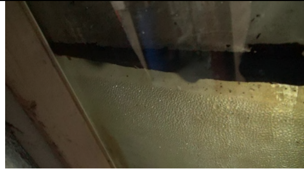
Figure C-o-50 Oil stuck to sides of tank at water surface
