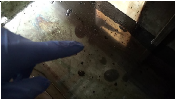
Figure C-o-23: AHS R5 S4 Oil blobs sunken to tank floor
