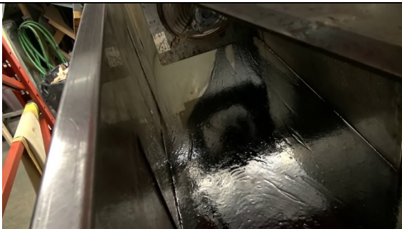
Figure C-o-318 WCS R5 S6 Hold-up on N side
