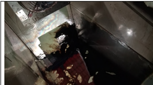
Figure C-o-32: ANS R3 S2 Oil slick temporary hold-up at fan
