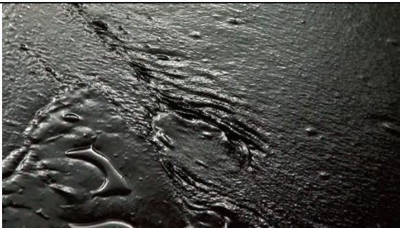
Figure C-o-324: WCS R6 S7 Weathered oil on N. side of tank
