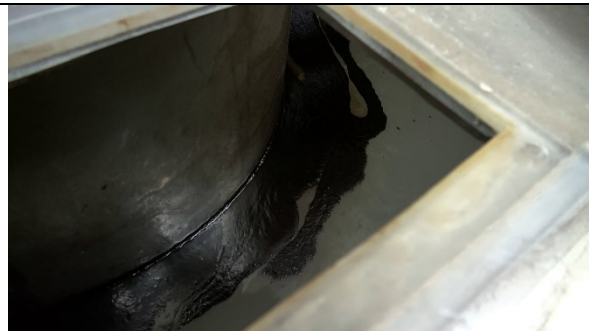
Figure C-o-319 WCS R5 S6 Oil along E side wall
