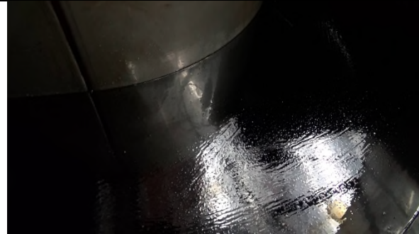
Figure C-o-259: SYB R2 S 1 Good oil coverage and circulation
