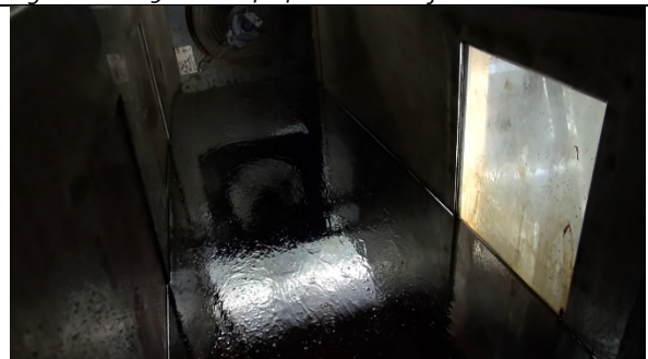
Figure C-o-231 MSW R4 S7 Final oil slick condition
