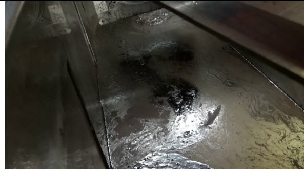
Figure C-o-81: CHV R3 S7 Hold-up between fan and thruster
