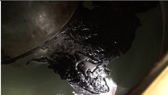
Figure C-o-236: MSW R5 S4 Thruster turned down, oil now flowing again
