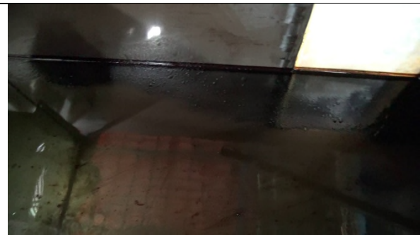
Figure C-o-94: CLB R1 S8 Oil layer at wall, none apparent on floor
