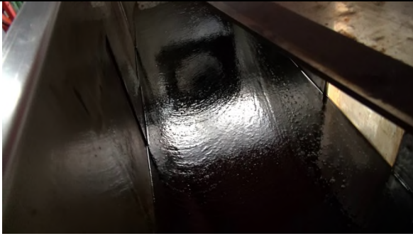
Figure C-o-188: LSB R4 S7 Oil hold-up between thrusters and fan
